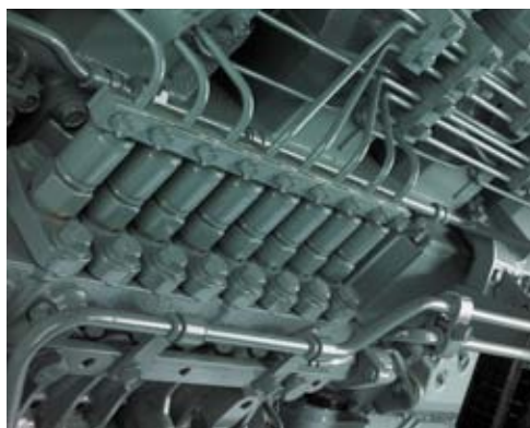
Diesel fuel lines
